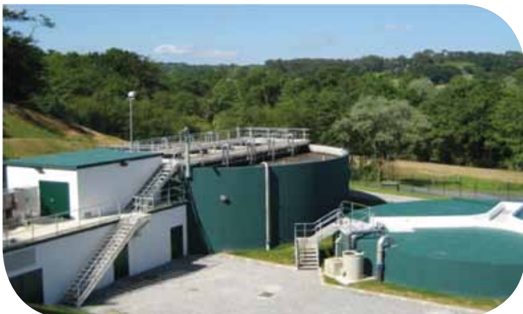
Bassussarry WWTP equipped with Alfa Laval MBR modules
